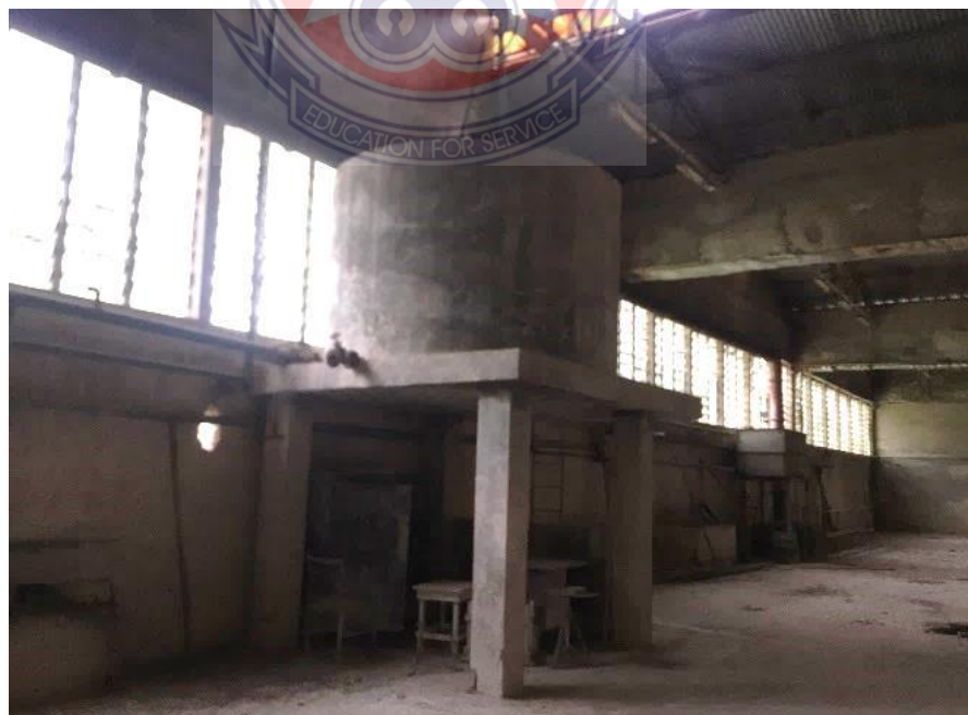
Fig 20: A water tank situated inside the factory
