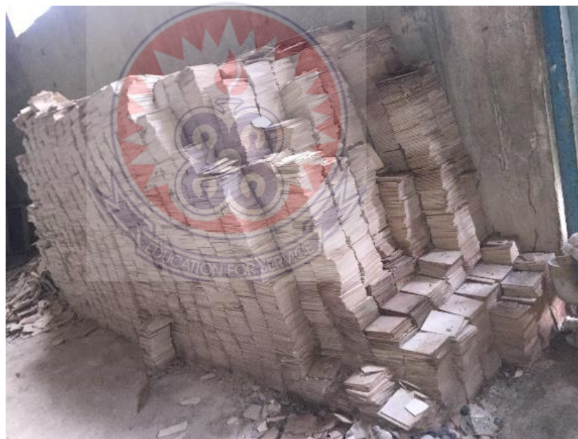
Fig 4: Pack of wall tiles found in the factory
