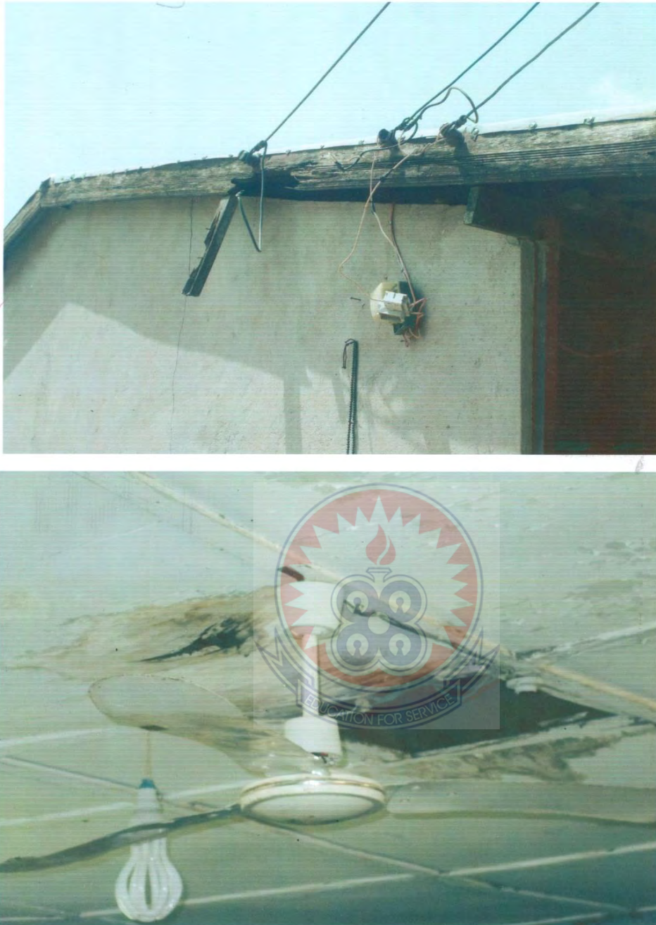
Figure 4.3 Exposed Electrical Cables and Fittings at the Senior High School
