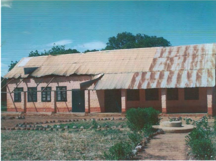
Figure 4.1 Leaking and Rusting of Roofed Members at Junior High School
