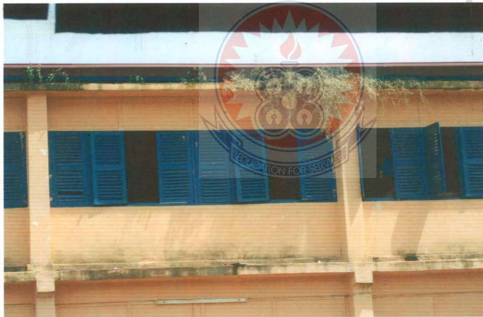
Figure 4.4 Dilapidated Structures at the Audit and National Service Office and the Senior High School
