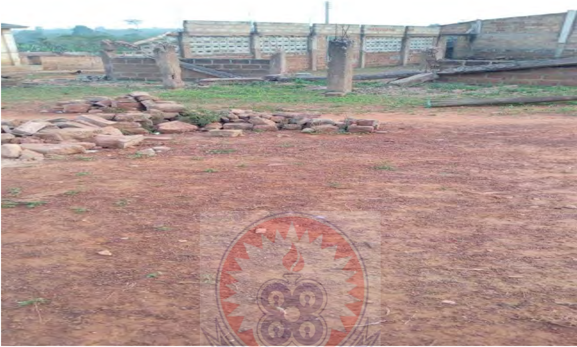
Figure 4.6: an abandoned construction work containing a lot of concrete, wood and steel waste s at the construction sites.
