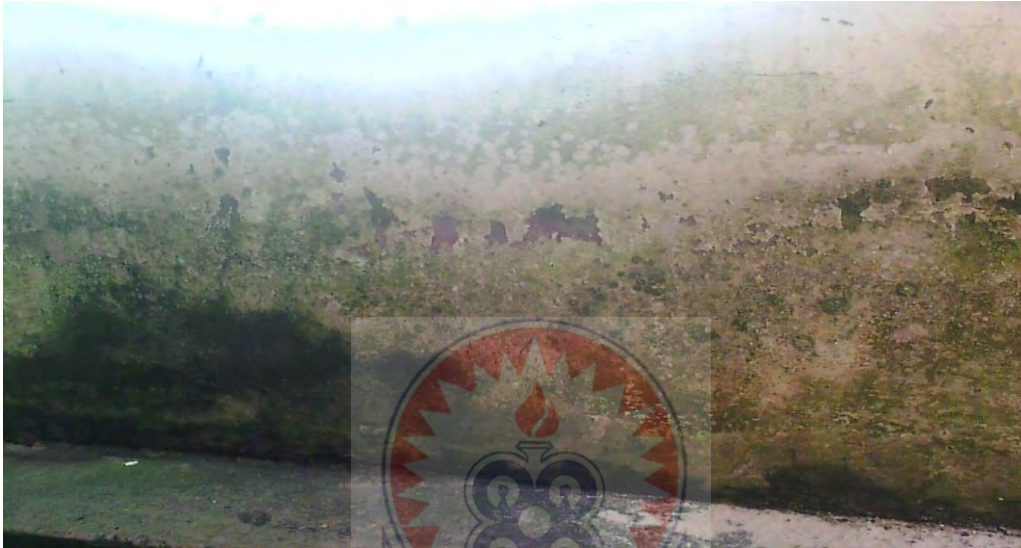
Fig. 4.3 Peeling off of Paints, Stains and patches of mold
