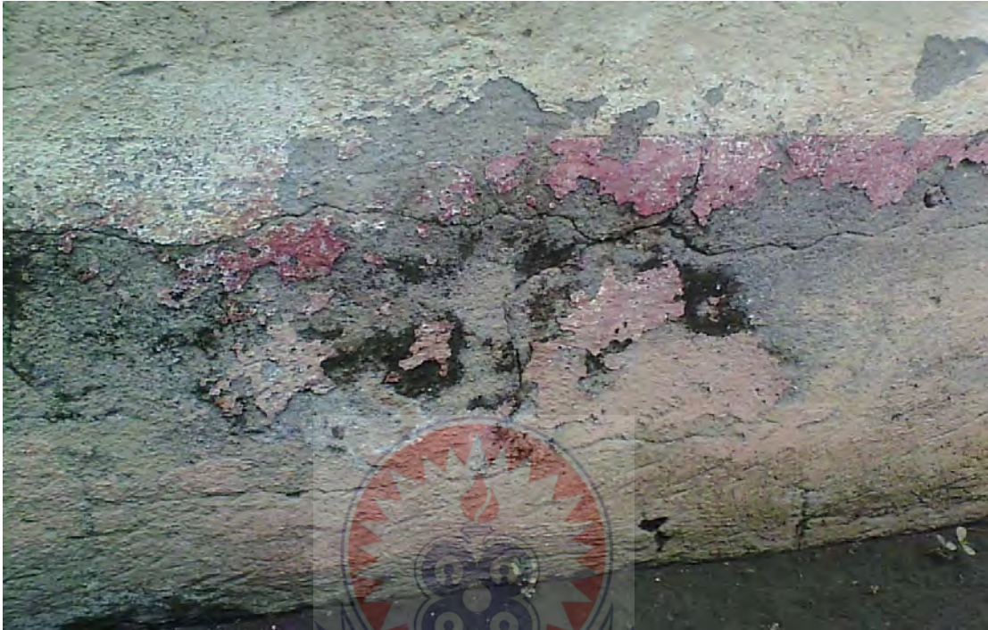
Fig. 4.1 Peeling off of paints, cracks, stains and patches of mold
