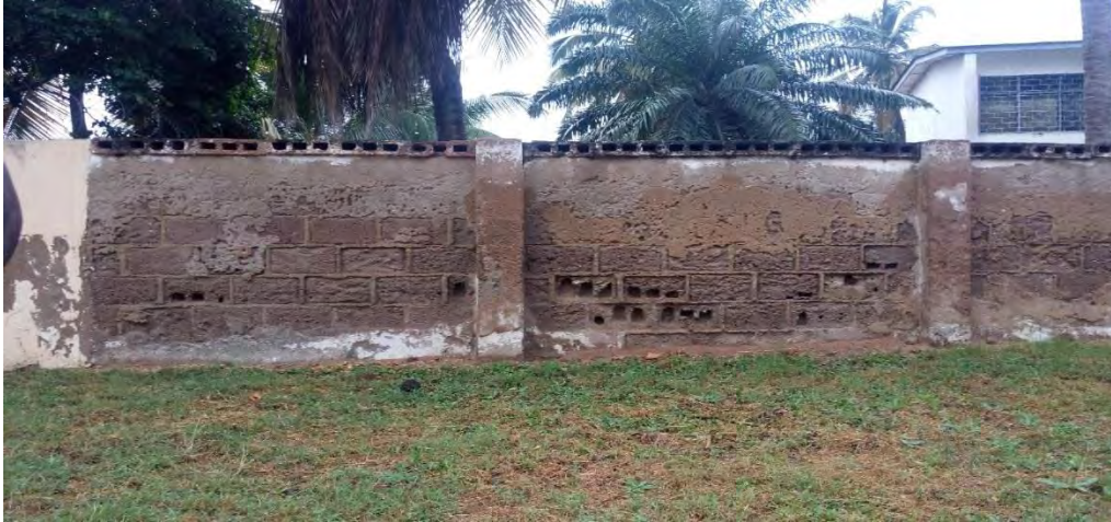
Fig. 4.4 Disintegration of building components and Wearing of plaster
