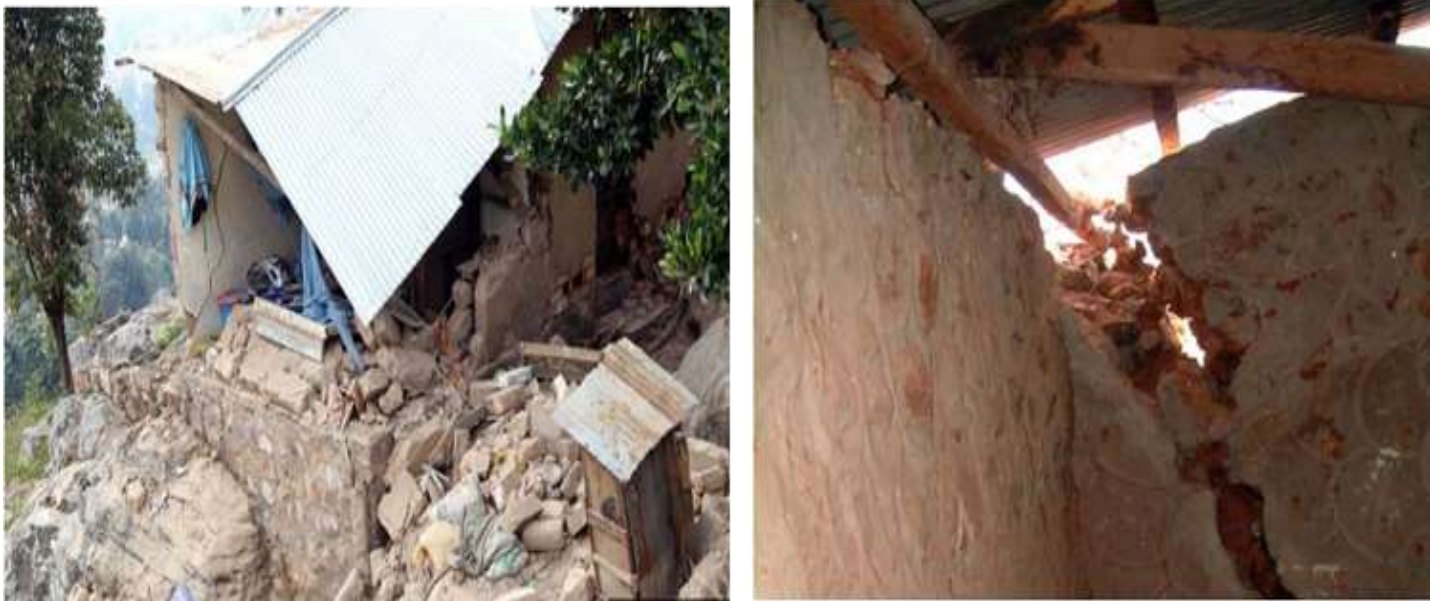
Plate 4.3: Aftermath of March, 2019 earth tremor at the hill top and last stop area Source: Field photo, 2020
