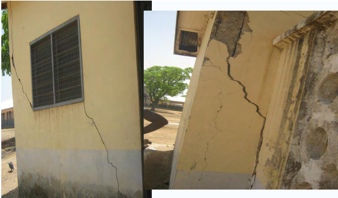
A 3-Unit apartment teachers' quarters at Ananteem in the Bolgatanga Municipality that has been abandoned due to several terrible structural cracks.
