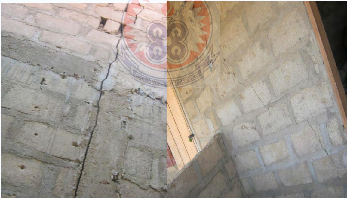
A building under construction that suffered serious structural cracks due to operational and/or constructional error at Sumbrungu in the Bolgatanga Municipality.
