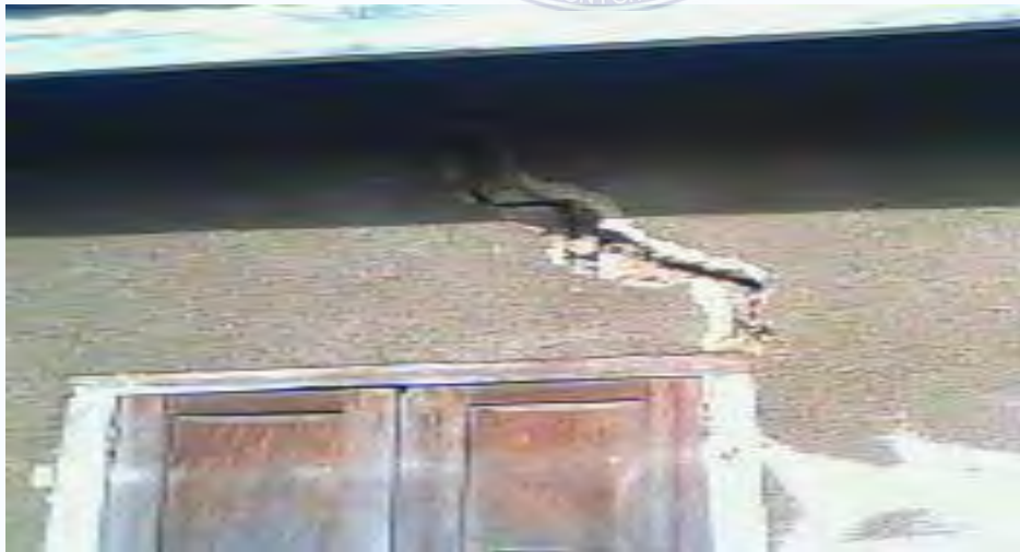
A building that cracked through a lintel which is an indication of operational error emerging from the lintel construction in the Sabon Zongo Residential Area.
