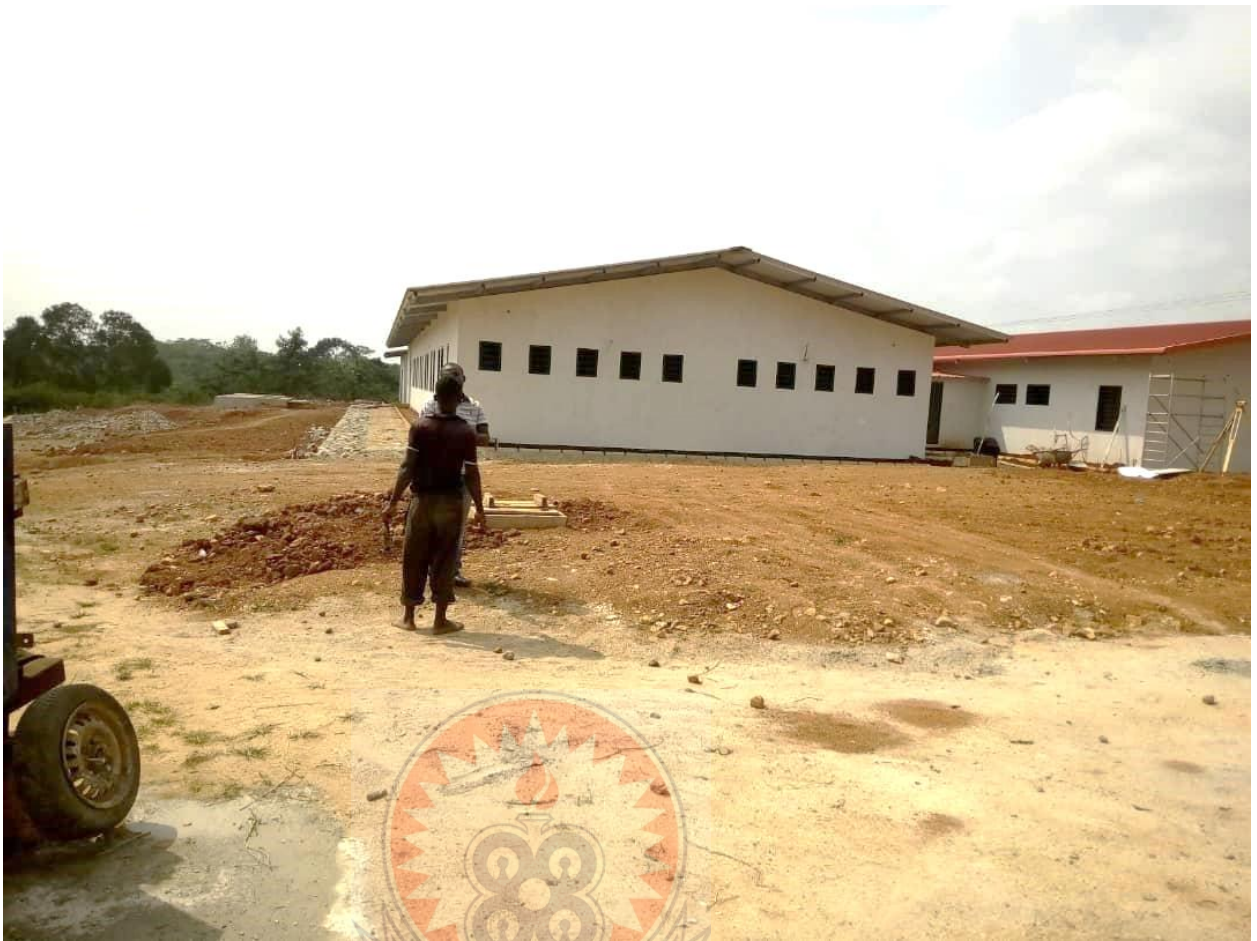
Figure 4.3: Plumbers Laying Soil Vent Pipes at a Poly Clinic at Gomoa (Dawurampong)
