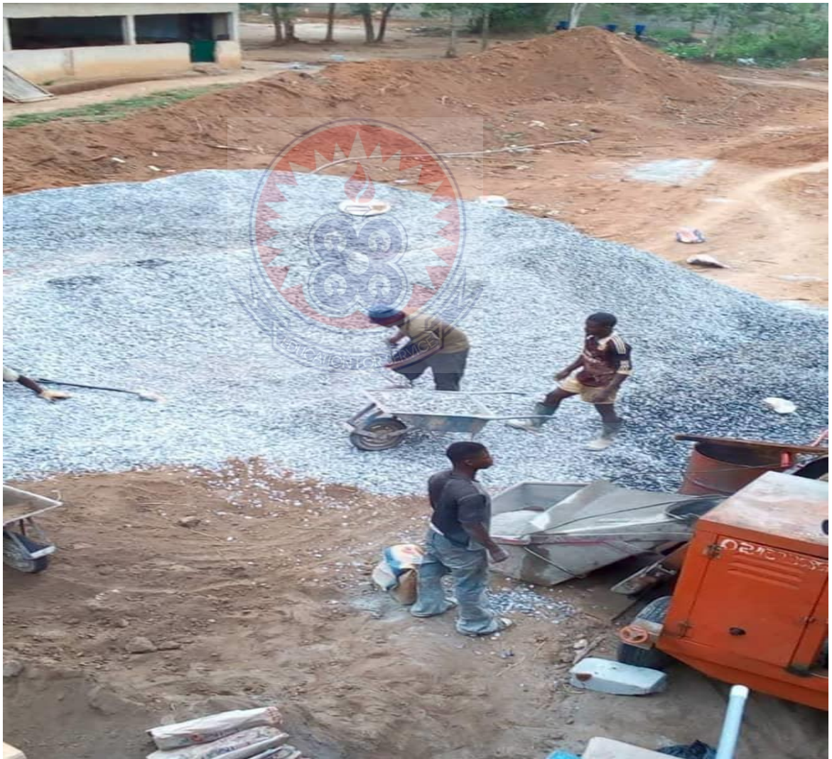
Figure 4.1 Mixing Concrete at the Site at Gomoa Senior High Technical School (Dawurampong)
