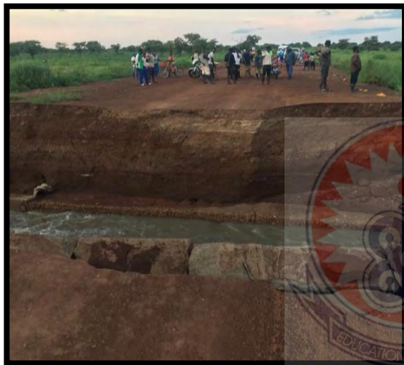
Major Road Cut-Off
