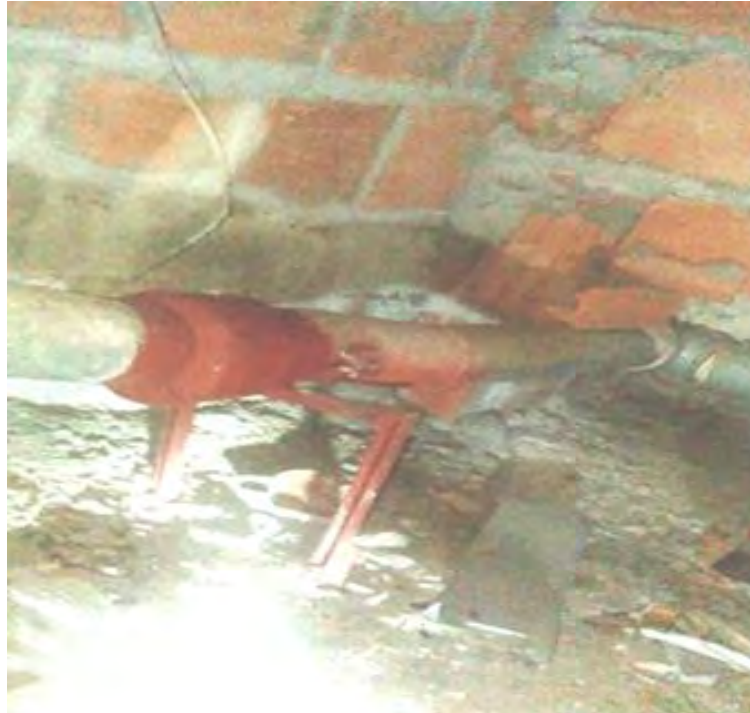
Figure 42: Leaked water in the Duct Space area as a result of a Broken Cast Pipe.
