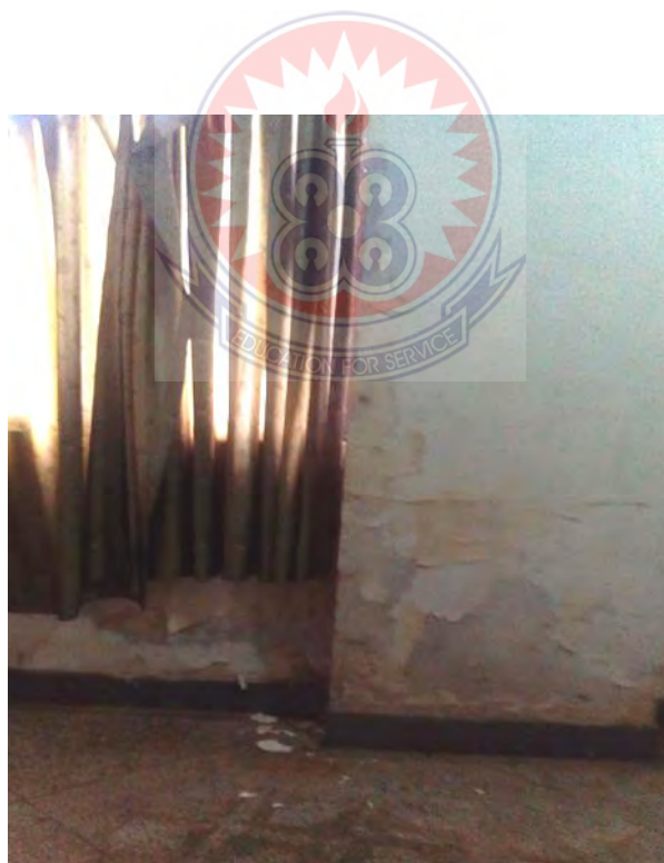
Figure 41: Oxidized wall of a changing room due to Broken Leaking Cast Pipe.
