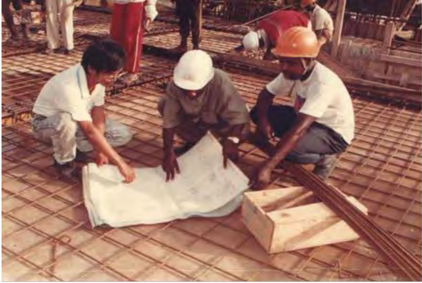
Figure 35: The Chinese Engineer in a discussion with the Ghanaian Engineer and the Foreman on the Project
