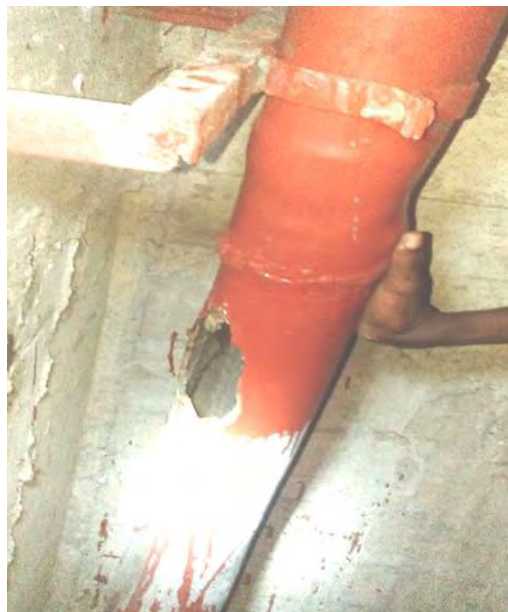
Figure 40: A Broken Cast Iron Pipe
