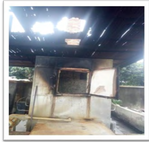
(b) Damaged roofing sheet by the incinerator
