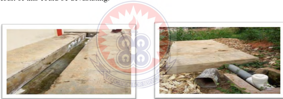
(a) Drain at Manhyia hospital
