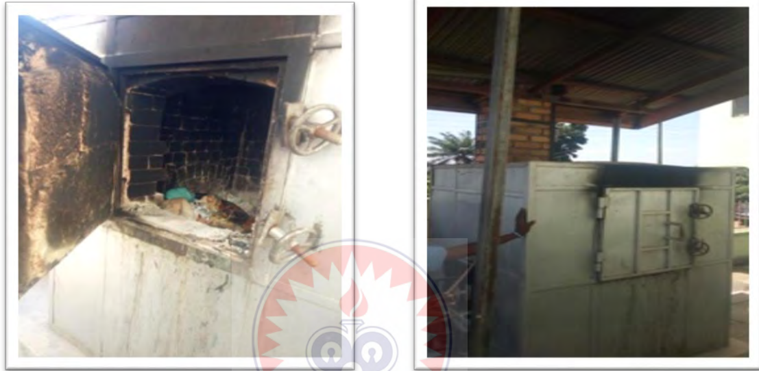
(a) Opened incinerator at Trust care hospital (b) Closed incinerator at Trust care
