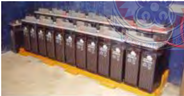
Figure 4.34: Battery mounted off the floor; source: Briganti
