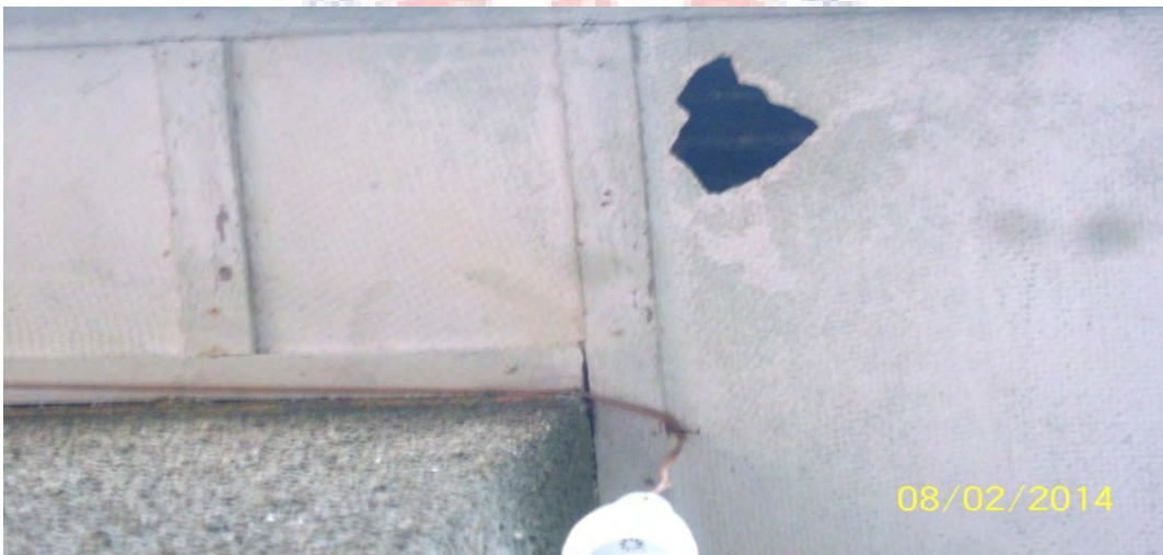
Fig. 4.19: Broken ceiling at GPS- Akim Akroso
