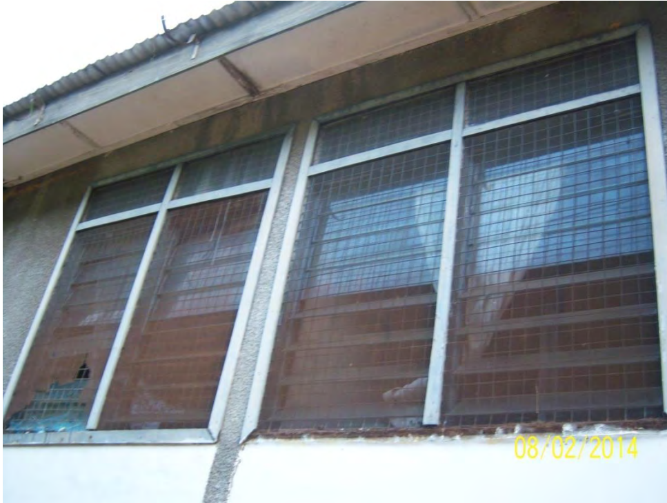
Fig 4.14b: Broken and tattered windows at GHS Nurses Quarters – Akim Akroso
