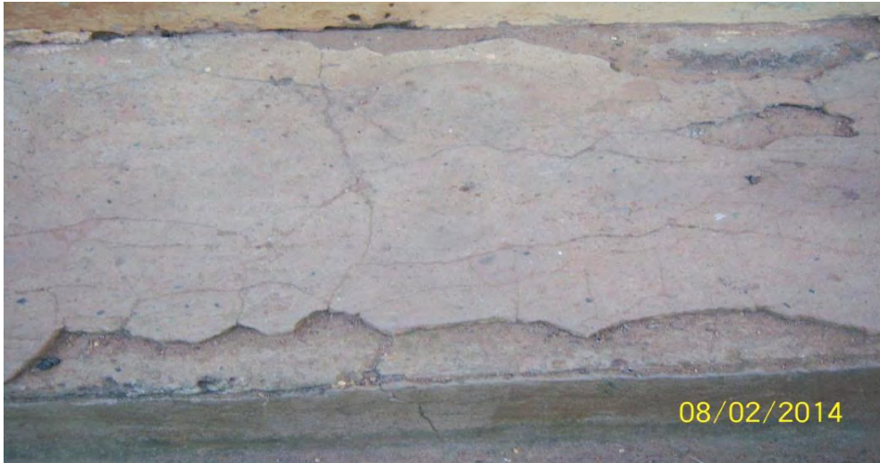
Fig. 4.18: Peeled off floor at GPS bungalows – Akim Akroso
