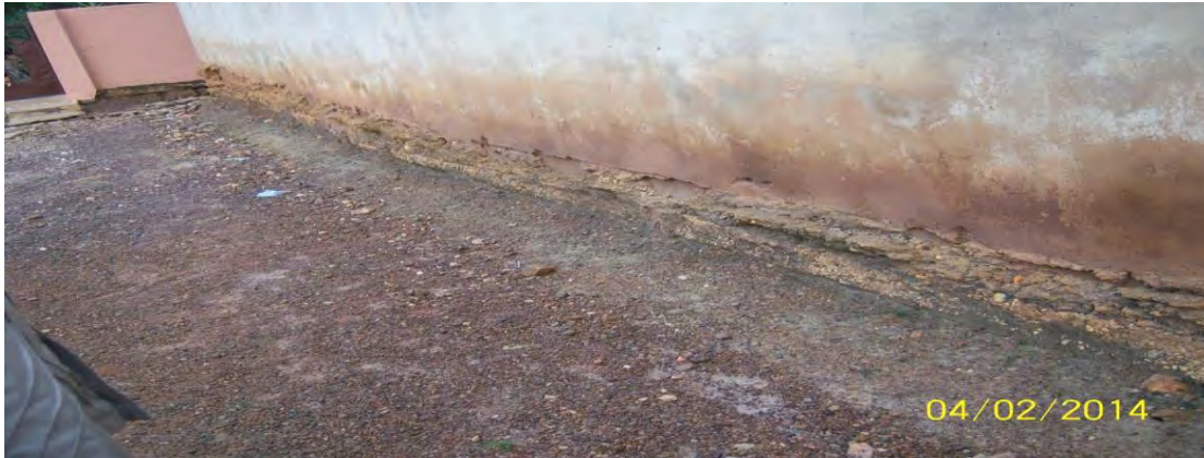
Fig. 4.10 Exposed foundations and faded paint walls at GHS Nurses Quarters – Akim Oda
