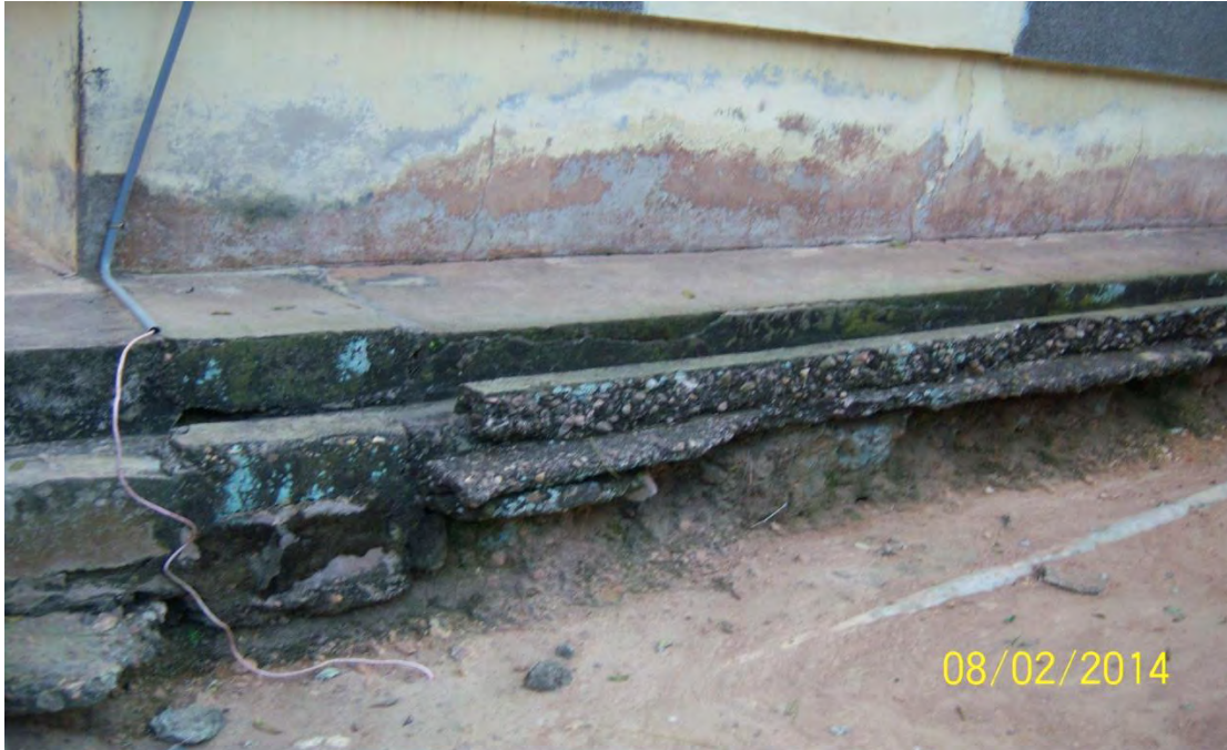
Fig 4.17: Eroded foundations at GPS Bungalows- Akim Oda
