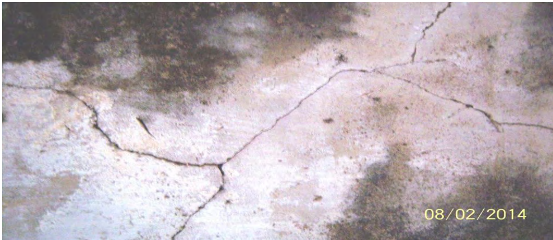
Fig. 4.15: Deep cracked walls at GPS bungalows – Akim Oda
