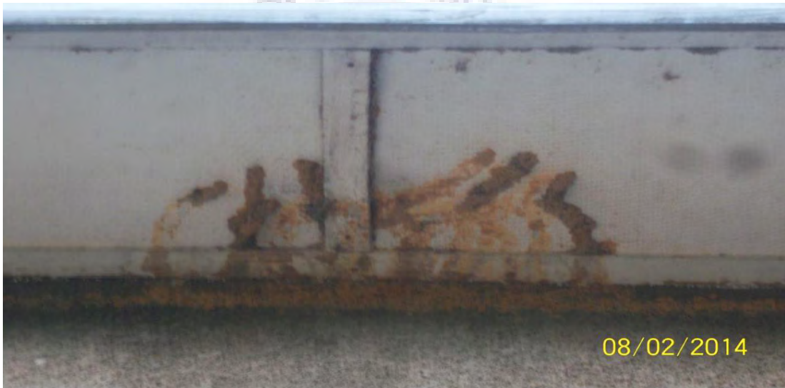
Fig 4.20: Roof leakage at Akroso SHS Bungalows– Akim Akroso
