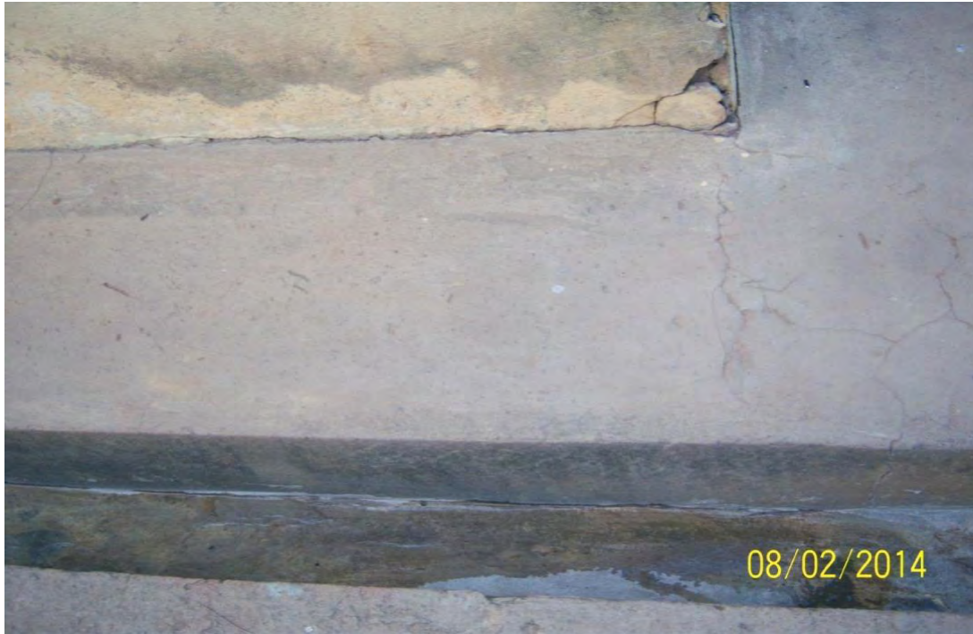
Fig 4.21: Peeled off floor at Akroso SHS Bungalows – Akim Akroso
