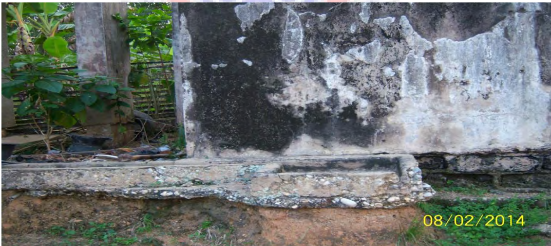
Fig 4.16: Fungal- infested wall at GPS Bungalows – Akim Oda
