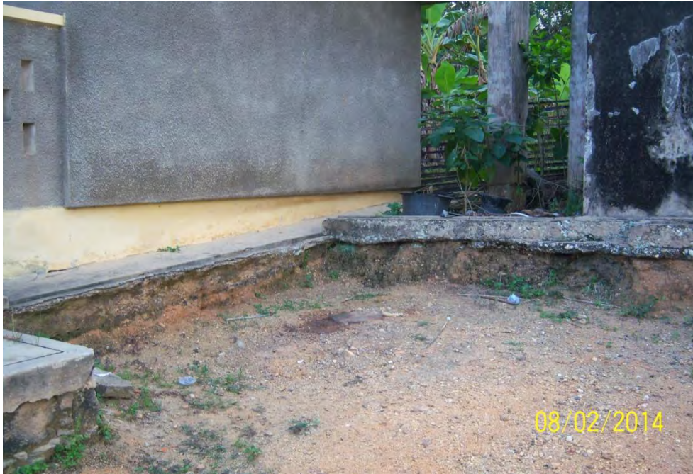
Figure 4.13: Foundation – Hanging and exposed at GHS Nurses Quarters – Akim Akroso
