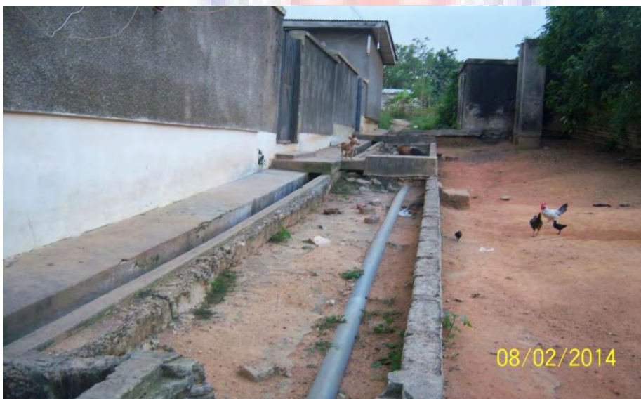
Figure 4.11: cracked and eroded gutters at GHS Nurses Quarters - Akim Oda
