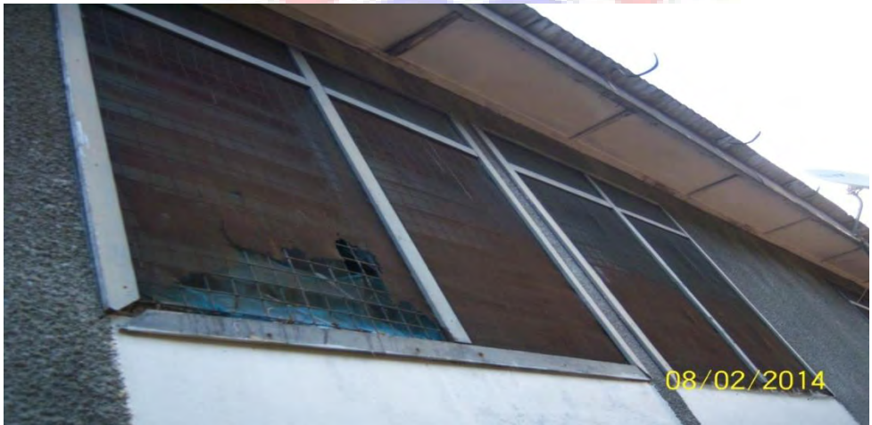
Fig 4.14: A Broken and tattered windows at GHS Nurses Quarters – Akim Akroso
