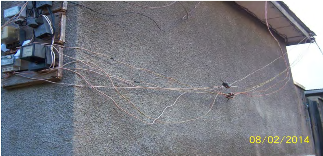
Figure 4.12: Faulty electrical system at GHS Nurses Quarters - Akim Oda
