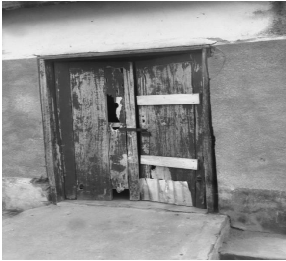
Rotten Doors Frames and Lid at Saboba District Assembly
