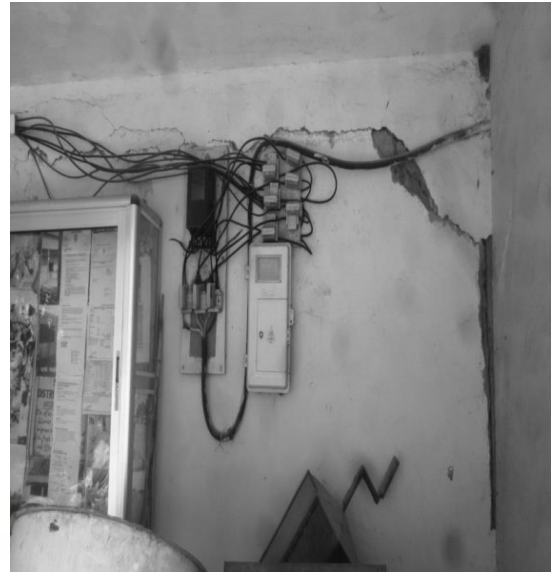
Figure 4.39 Exposed Electrical Cables at Saboba Medical Centre/GHS
