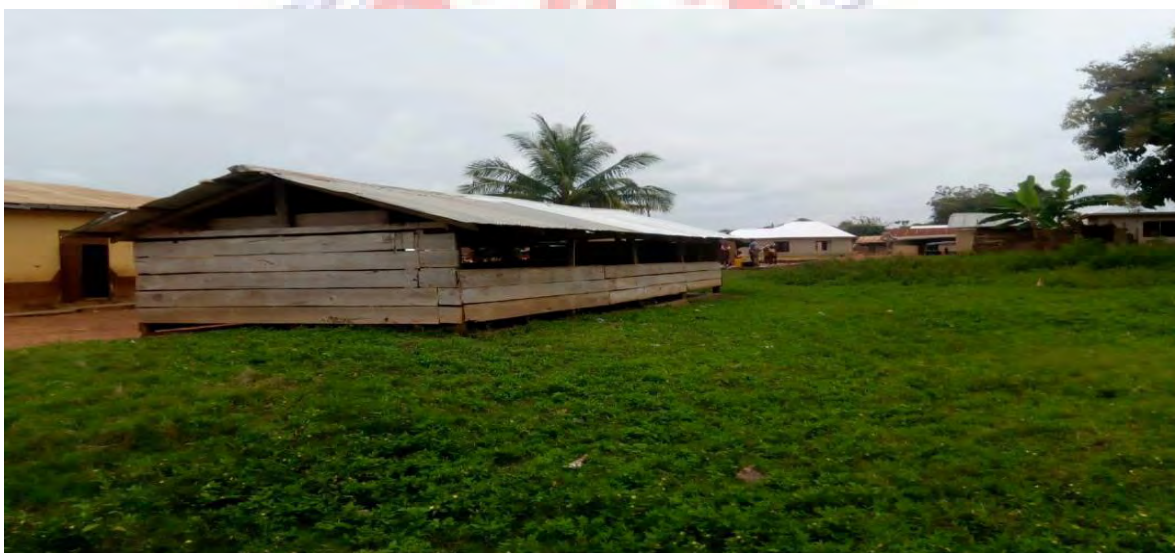
Figure 5: Dilapidated building for one of the preschools (public school)
