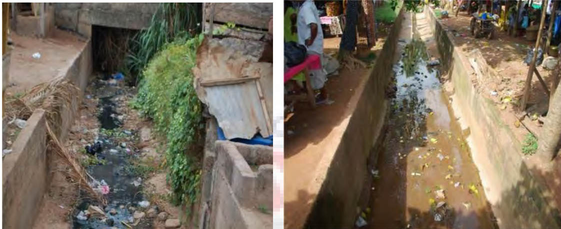
Figures 4.2 & 4.3: Solid waste dumped in open storm drains
