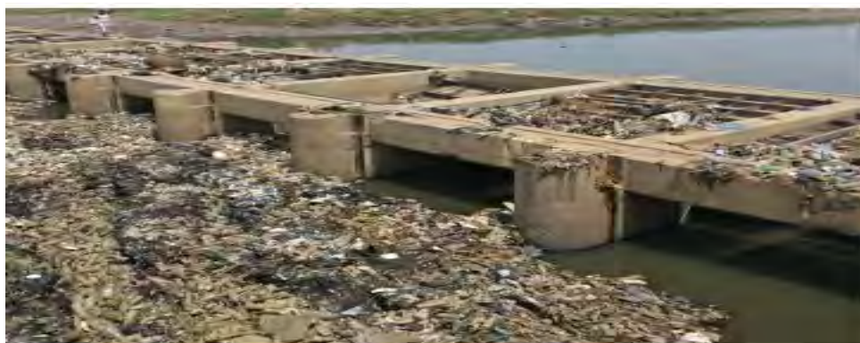
Plate 1: Pollution to the lagoon from the gutters at Traffic light and HFC bank Source: Field Survey (2019)
