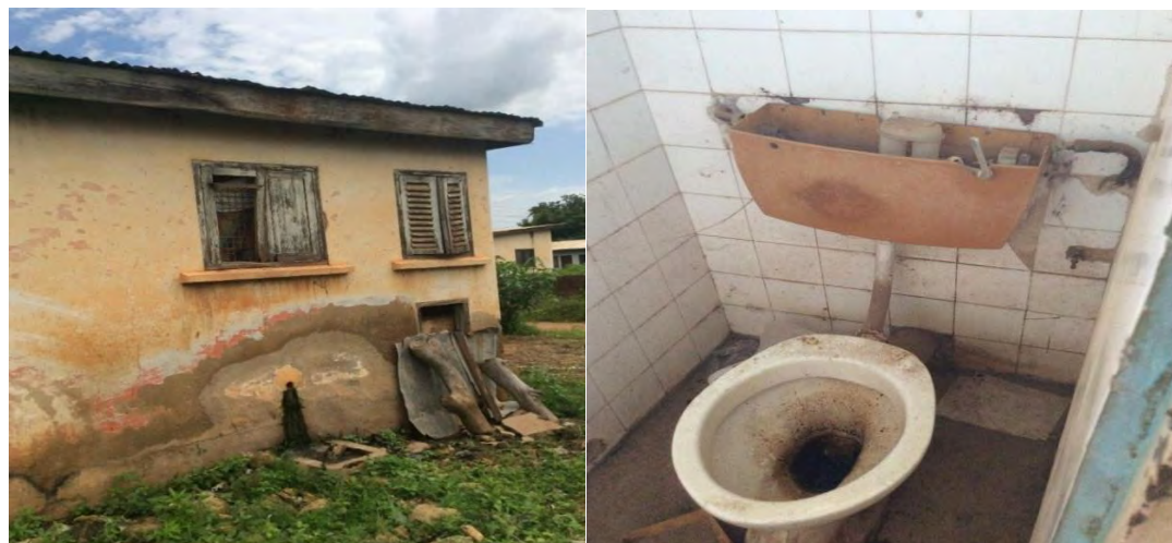
Figure 4.6: Pan Latrine and Non-functional water closet facility
