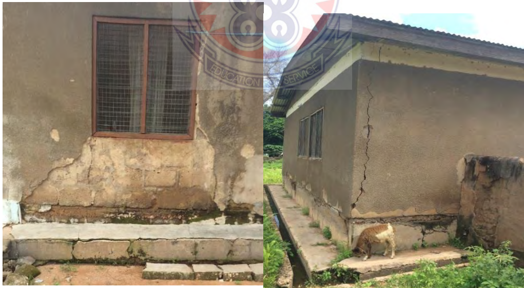
Peeled-off plaster & Crack on walls due to old age and poor maintenance of buildings
