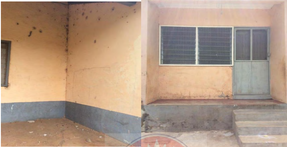
Painting; Dirty and Faded walls
