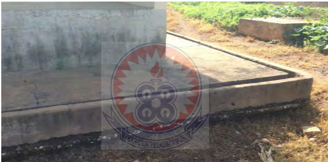
Figure 4.3: Exposed/hanged foundation due to erosion
