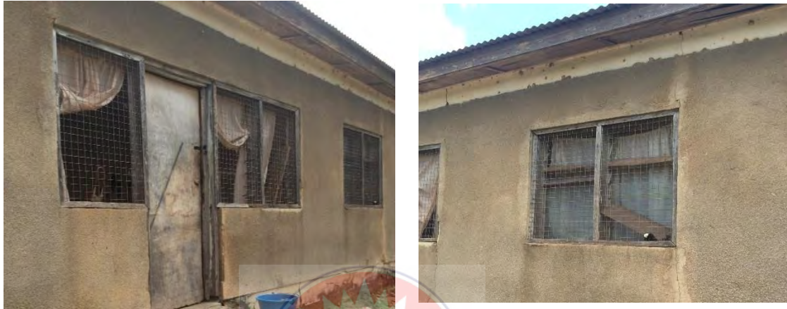
Figure 4.5: Missing louvre blades and weak wooden members (door & window frames) due to poor maintenance practice.
