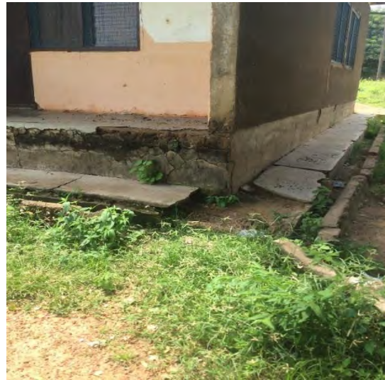
Weak floor & foundation due old age & lack of maintenance of buildings weak structure
