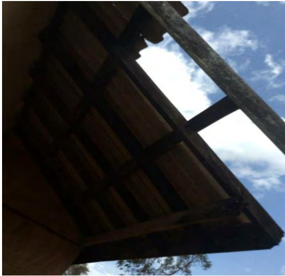
Roof: Partly ripped off
