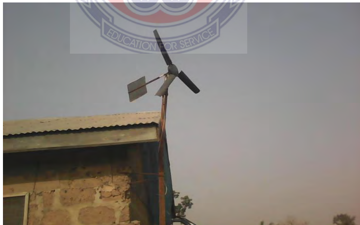
Figure 3.12: Shows the generator (wind turbine) mounted on a pole for testing.
