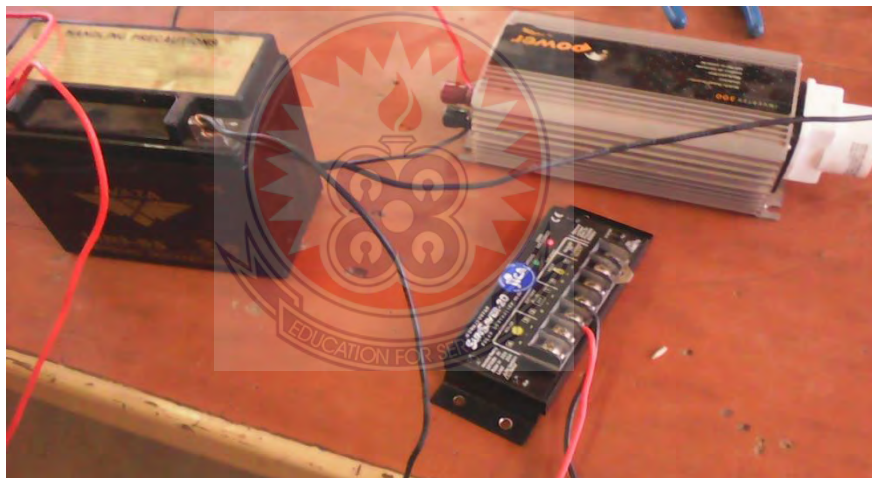
Figure 3.10: Show the electronic components connection. Charge controller connected to 15 plate 12V lead acid battery and to DC / AC inverter.
