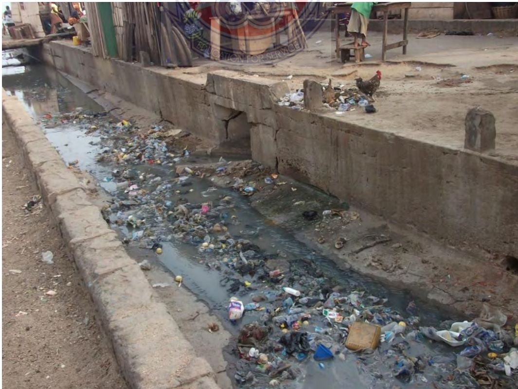
Fig. 4.3: A Gutter at Wonsom market used as a Refuse Dump Site
