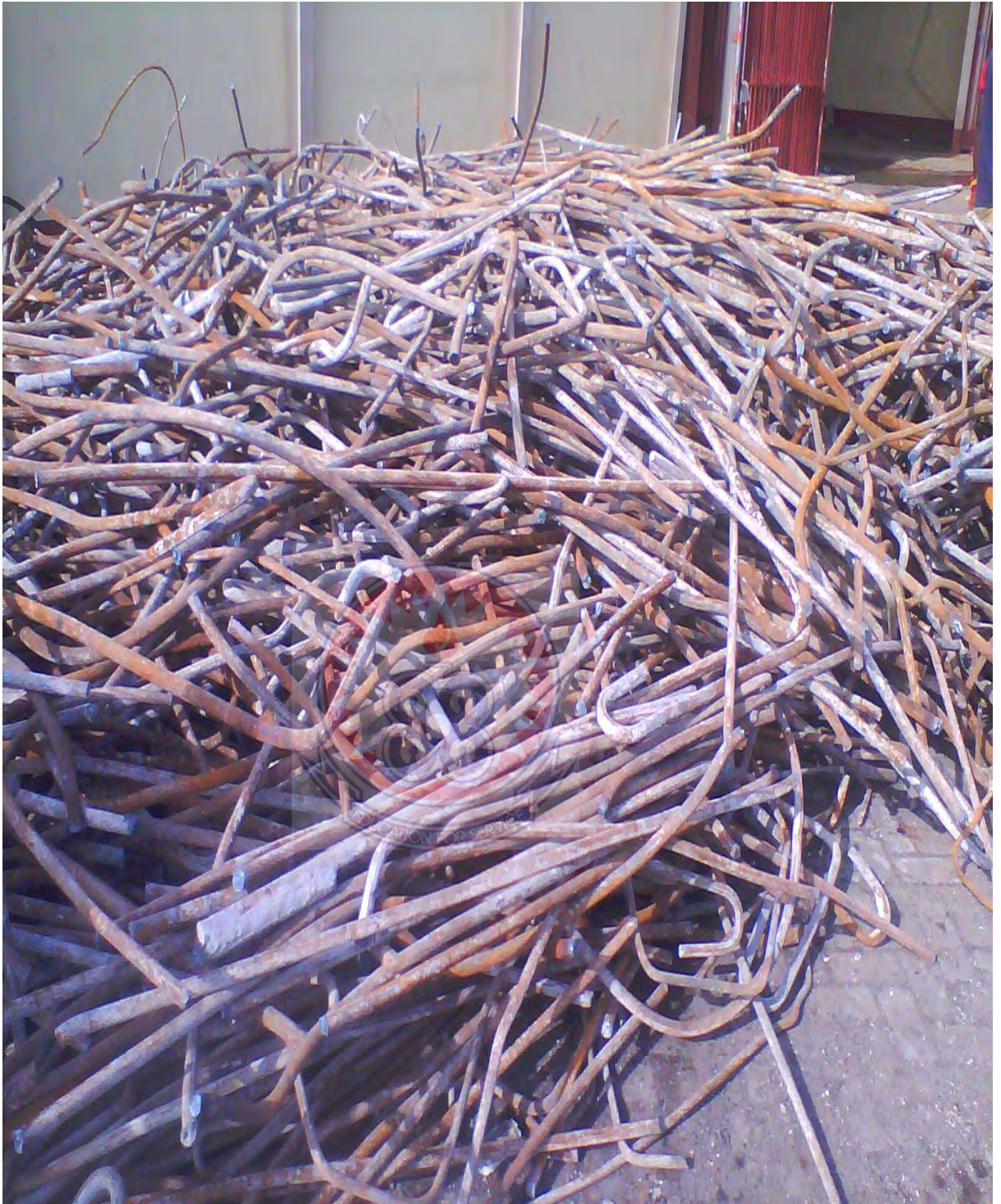
Waste Iron Rods on Site
