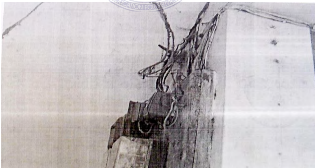
Electricity: Exposed Cables
