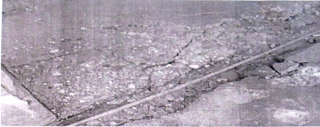
Cracked developed on concrete ground floor
