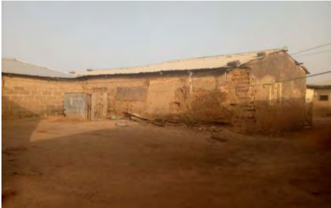
Figure 4.1: Dilapidated Housing Structure in Dondoli Community of Wa
