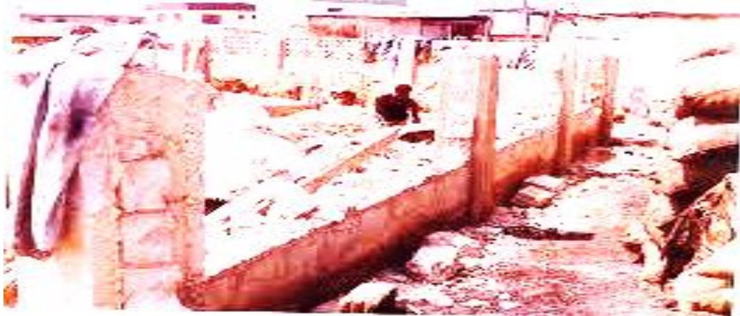
Figure 4.7. Private property demolished as due to land ligation at Kasoa-Central Region. Source (researcher's field data)
