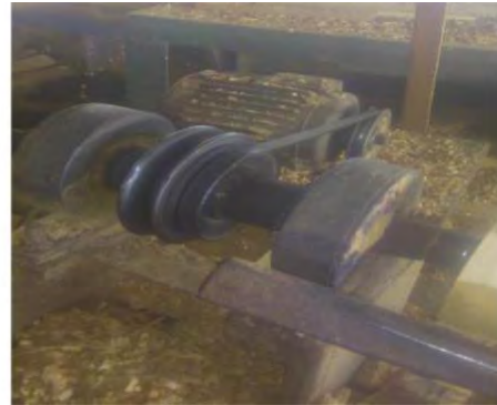
Figure 4.5: Wood mortiser guard enclosing the chains and driving mechanisms.
