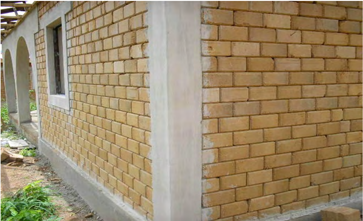
Fig 2.6 Interlocking / hydrofoam Masonry blocks at the finishing stage of a housing project
