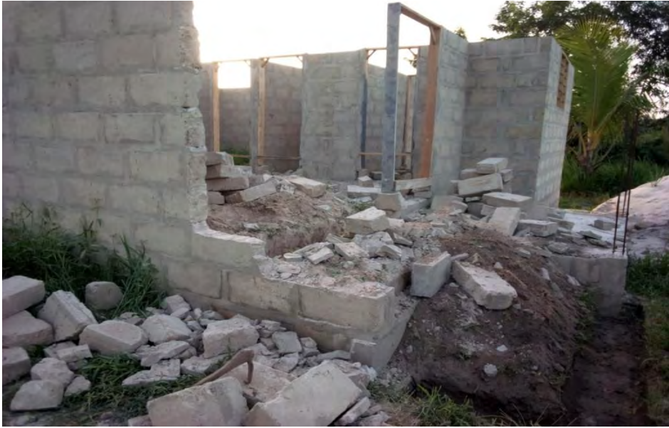
Figure 4.5 show the destruction of building due to made up ground at Oyoko
