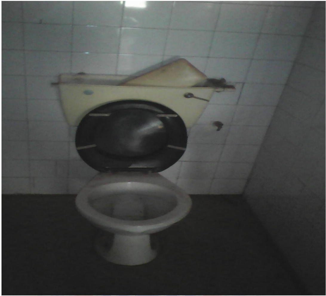
Figure 4.14: Broken-down Water Closet of students hostel at U.D.S Tamale Campus.
