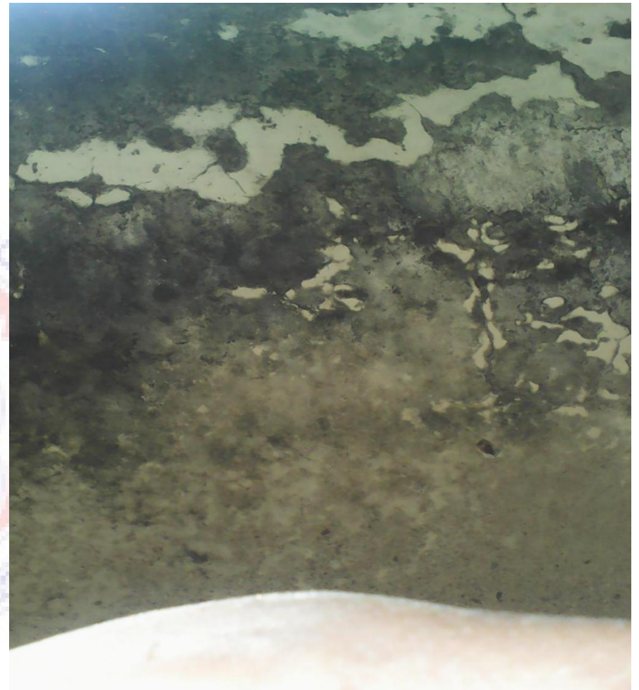
Figure 4. 5 Discoloured Paint of teacher's quarters building at Dabokpa Technical Institute
