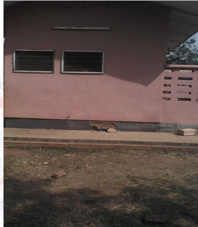
Figure 4.10: Exposed Foundation of nurses' quarters No. 1 Tamale Teaching Hospital.
