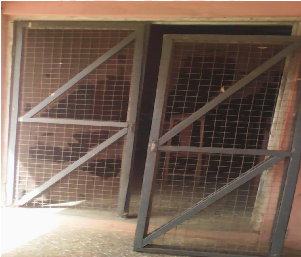
Figure 4.11: Broken Door of bungalow No. 2 at U.D.S Tamale Campus.
