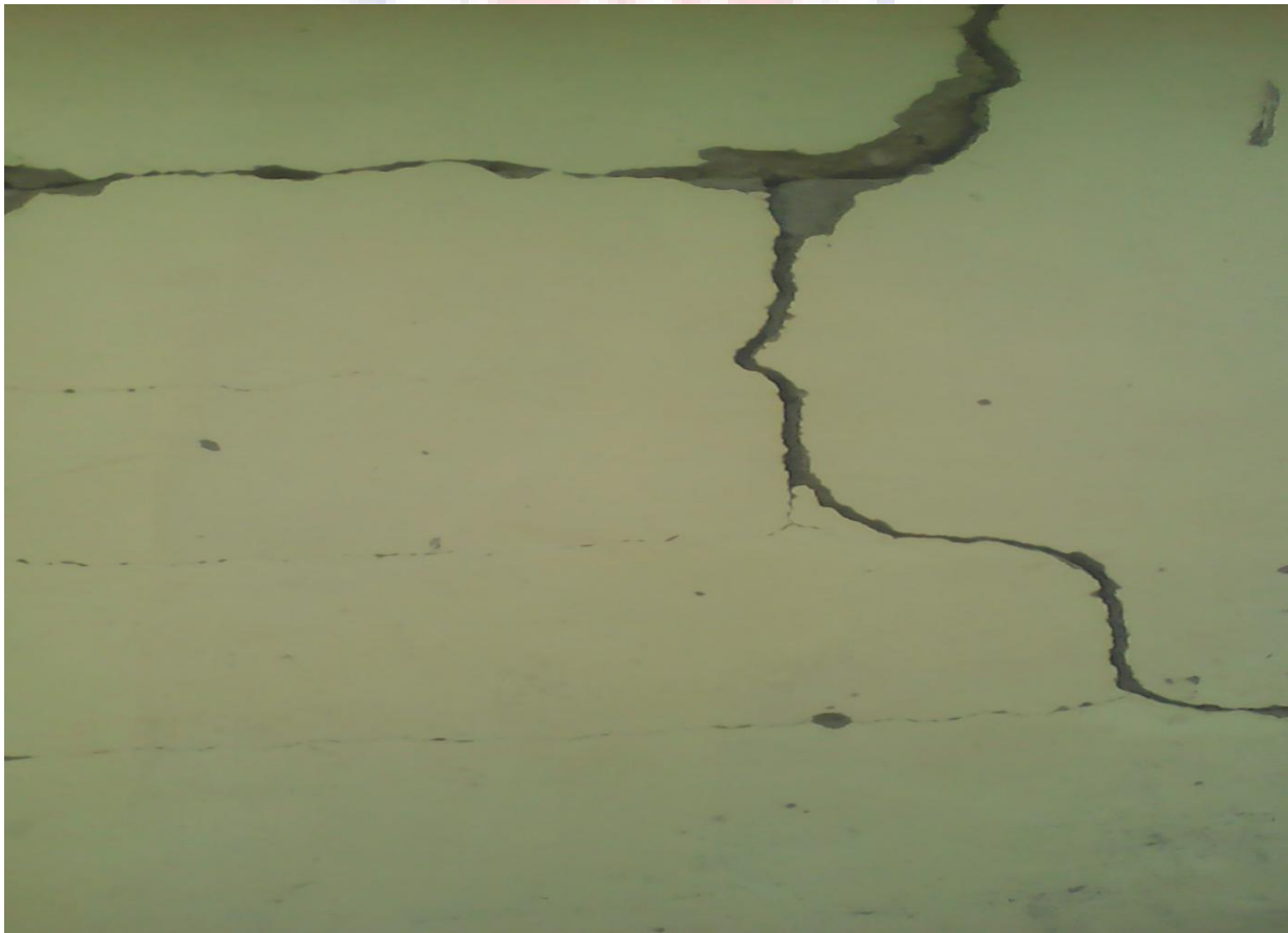
Figure 4. 8 Crack on wall of nurses' quarters No. 2 at Tamale Teaching Hospital.
