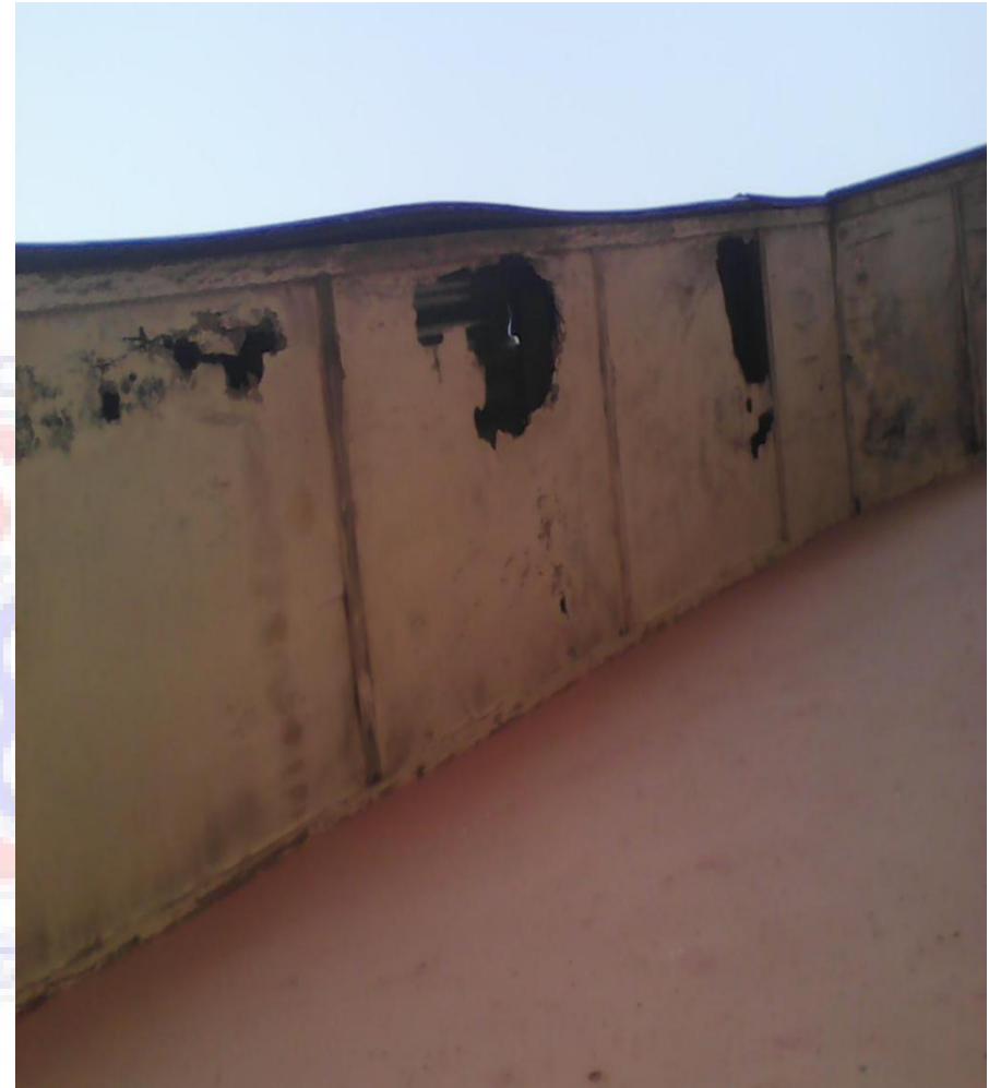
Figure 4.13: Defective Ceiling of maintenance workshop at U.D.S Tamale Campus.
