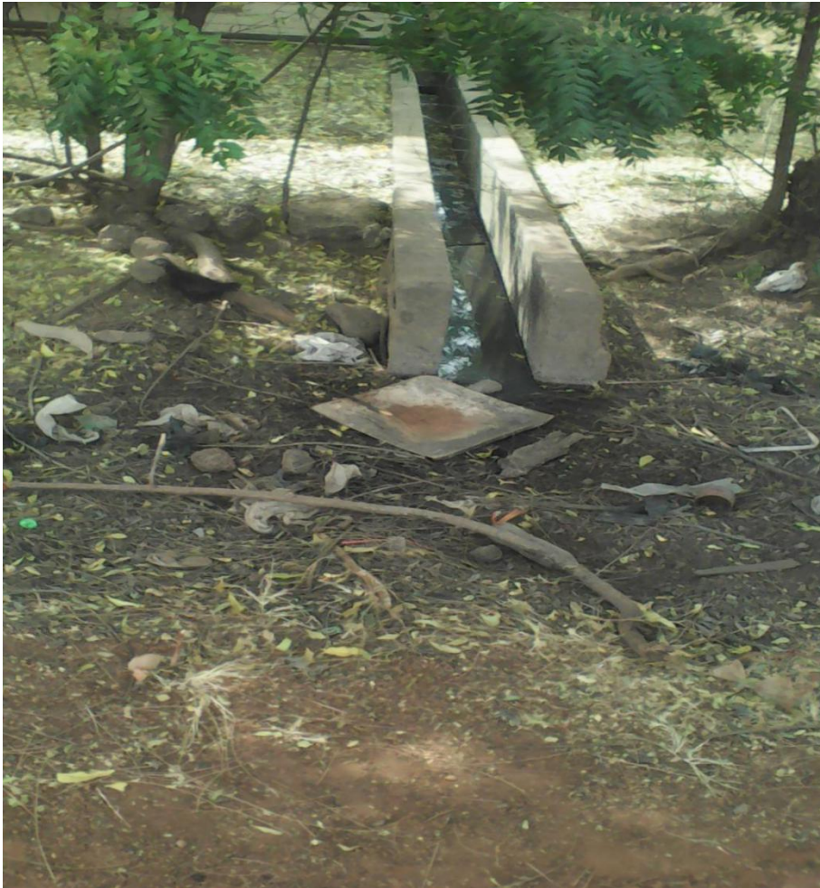
Figure 4.12: Choked Drainage System of Lecturers bungalow No. 3 building at U.D.S Tamale Campus.
