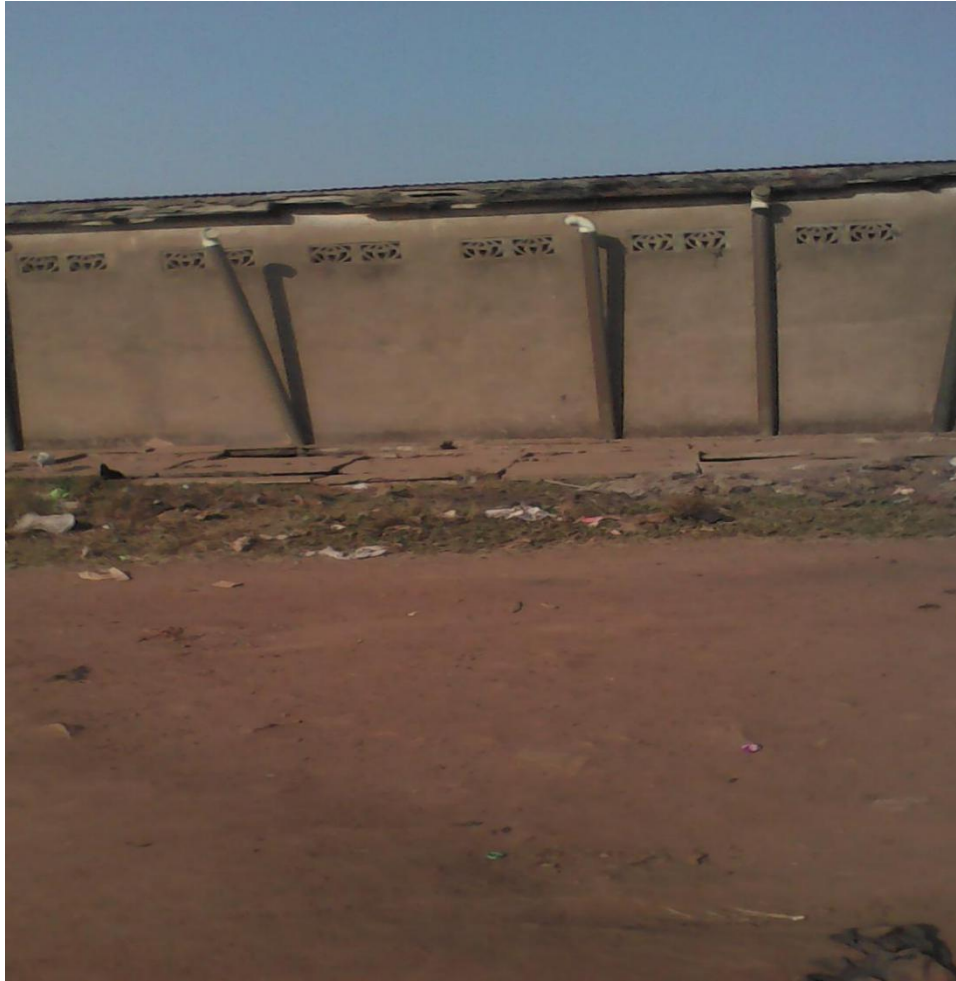
Figure 4. 4 Rotten Facial Board of toilet building at Dabokpa Technical Institute
