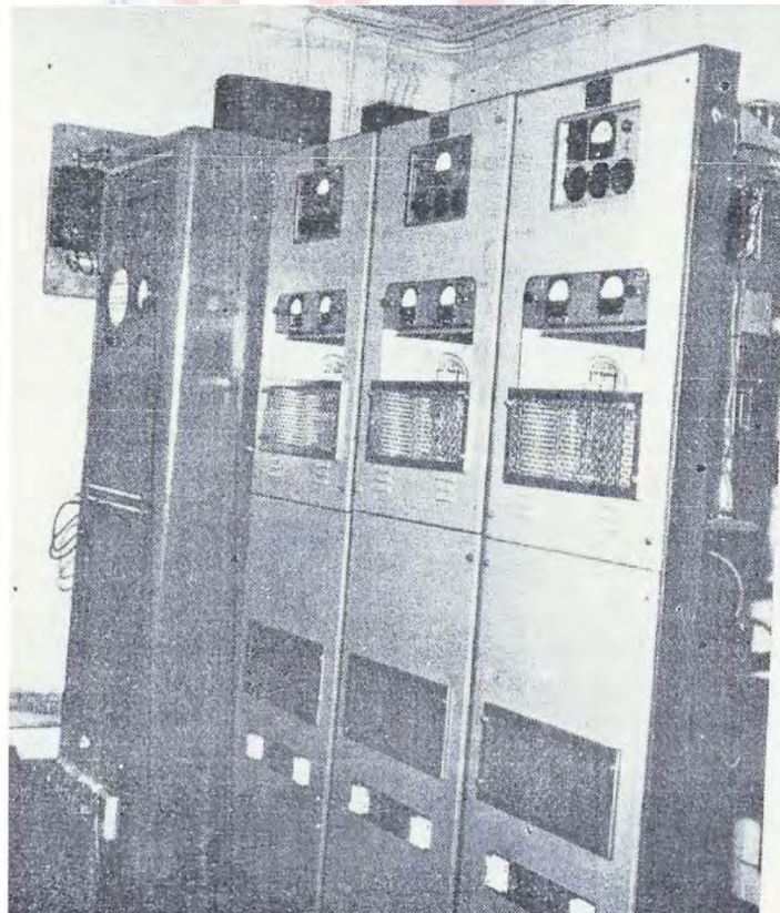
Figure 4.11: Audio frequency power amplifiers used in the Cape Coast Regional Station (Source: GBC Reference Library, Accra, 2017.)
