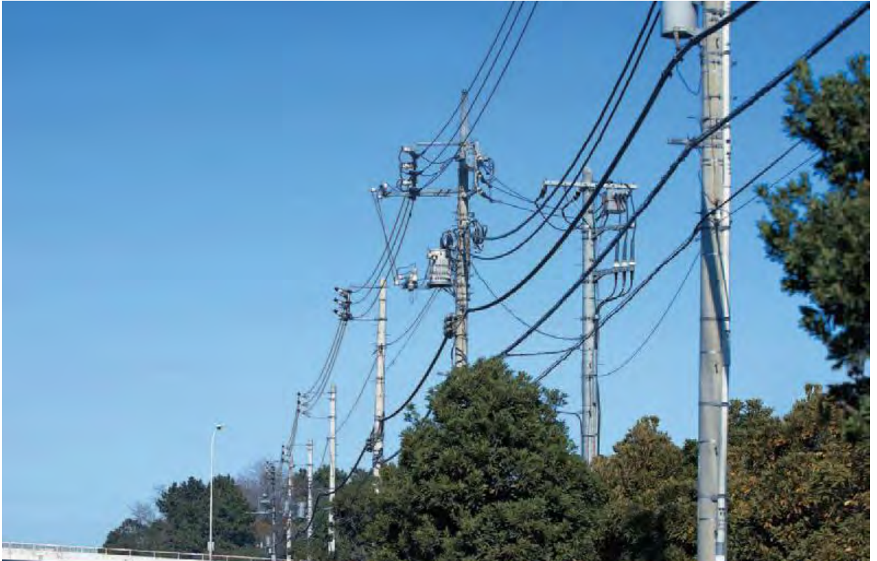
Figure 2.3: An overhead cable
